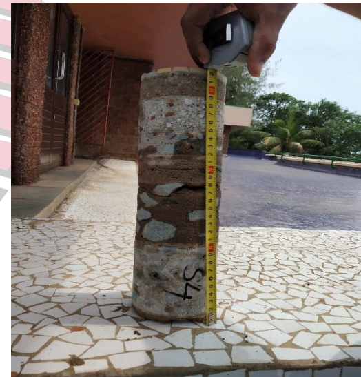
Repeated repairs/overlays on roof elements (thickness increased from 10 to 30+ cm)
